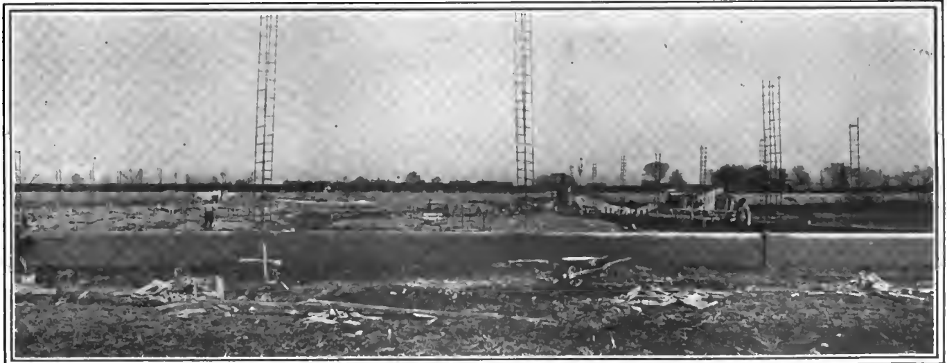
Laying the foundations for the new steel and concrete plant of the Chandler Motor Car Co., Cleveland, O.
